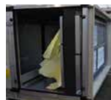
Combined Filter Section
